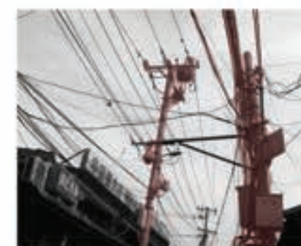
4. Power line mess
