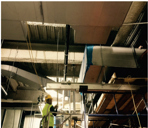
9 ph (05-31-2017) 4 th floor – outside Theater Wall. 64x24 SA duct installation in progress, miscalculated height of preexisting pipes
