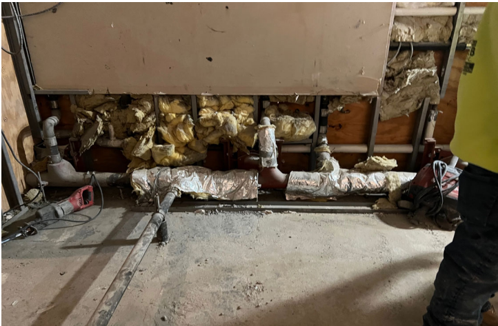
North side of ex PDR– waste pipes
