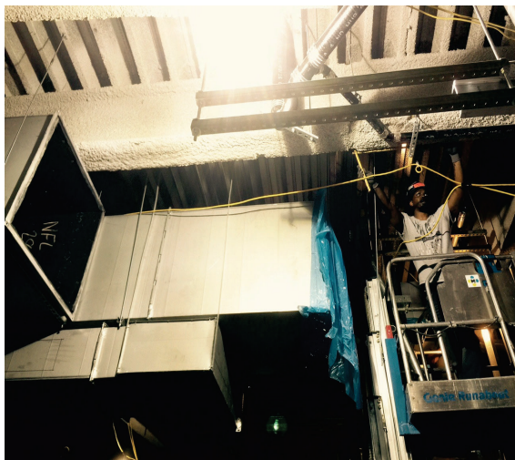
5 ph (05-19-2017) 4 th floor – Issues with preexisting pipes at the “West corridor” outside of the Theater, obstruction to ducts
