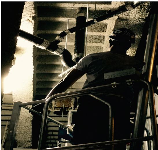
6 ph (05-19-2017) 4 th floor – Issues with duct passing on the “West Corridor”.
