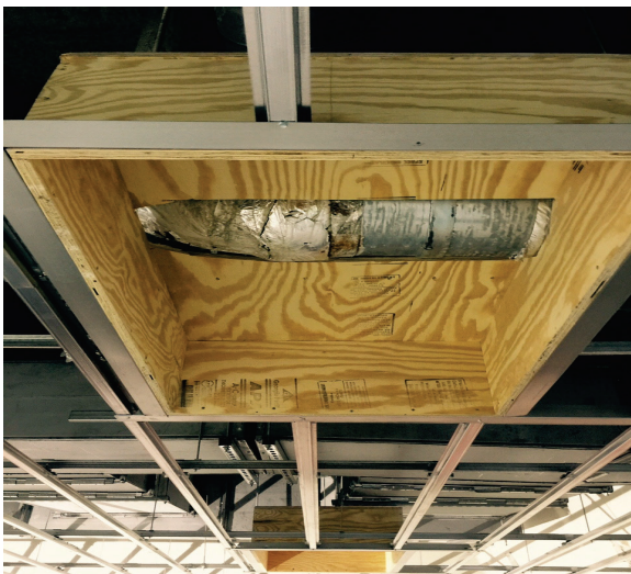
3 ph (07-17-2017)-Theater. warning ignored of preexisiting pipe conflict with speaker box.
