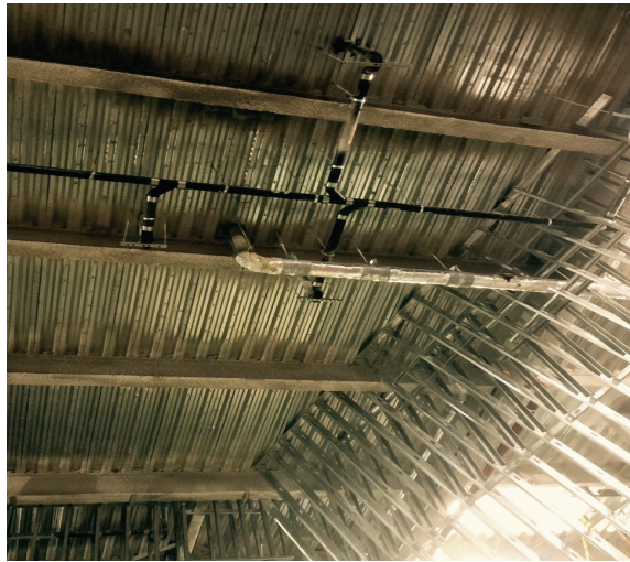
1 ph (04-14-2017) Theater North wall existing condition 9 inch thick pipe in conflict with mech duct installation & speaker box
