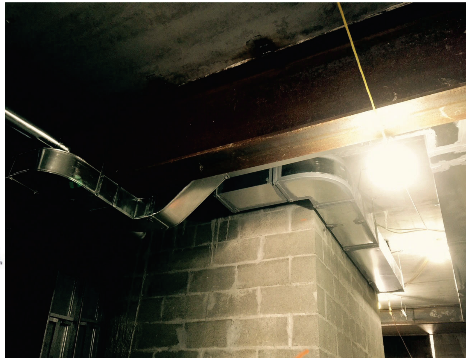
MECHANICAL DUCT DEVIATED TO LEFT CORRIDOR TO SUPPLY AIR TO SUPERS ROOM THIS SOLUTION WAS PROVIDED BY MARIA RENGAN UPON SITE VISIT
