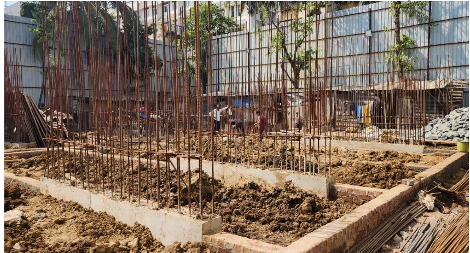
The foundation embeds flexible ground-floor use, designed for parking, play, or informal gatherings - reflecting how residents previously adapted shared spaces.
